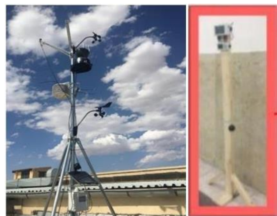
Figure 9. On the right side, The equipment placement inside the building. On the left side, The Hobo RX-3000 weather station [31].
